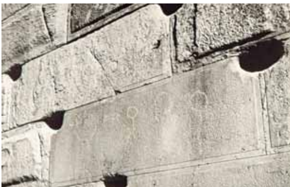
Fig. 3 A detail from the west façade of the tall stone platform that protrudes from one side of the Tall-e Takht or 'Throne Hill'. Note especially the delicate point stippling in the raised central panels and the neatly drafted edges visible on a number of the finished ashlar. Photo: D. Stronach.
