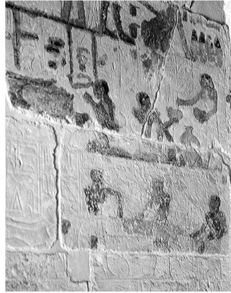
Fig. 4. The present condition of the wall painting of fig. 3 (in situ photograph by Aris Gerontas)
