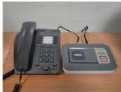
Data Center Communication
